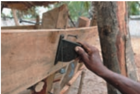
Figure 2 A plumb bob is a relatively large mass hung on a cord. To be sure that fence posts, walls, door and window frames, and strips of wallpaper are vertical, a construction expert or an interior decorator suspends a bob to check whether the vertical lines are parallel to its cord. To obtain a horizontal line, a 90^\circ angle can be drawn from the vertical.
